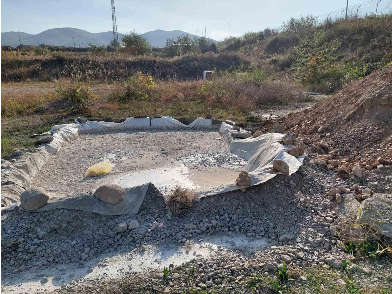
Washout pit covered with geotextile
